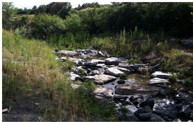
Photograph 8-8. Proactive stabilization at McMurdo Gulch, constructed with little disturbance to the existing channel.
