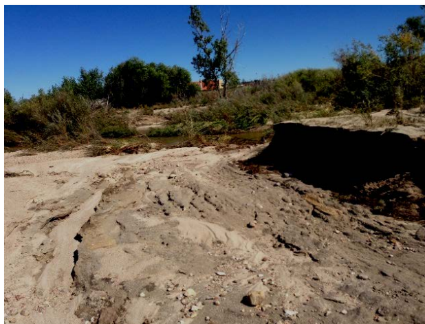
Photograph 8-9. Degradation in a channel.
