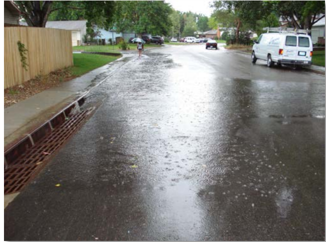
Photograph 7-6. Weir performance decay can be observed in this picture as flow appears to enter only the first two inlets while exceeding the height of the upstream curb.
