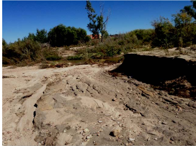
Photograph 8-9. Degradation in a channel.
