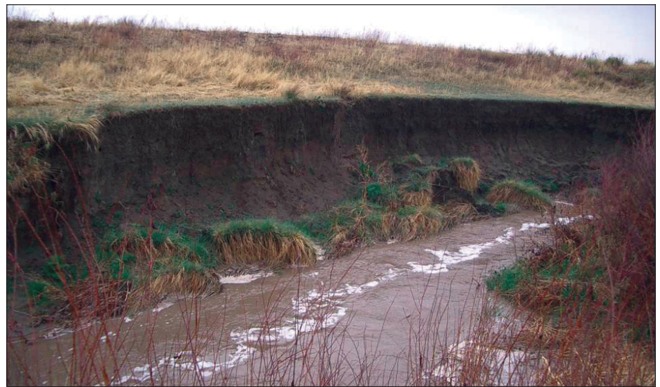
Figure 5. Prior to the project, Cottonwood Creek was deeply incised and actively eroding, conveying phosphorus-laden sediment to Cherry Creek Reservoir.
