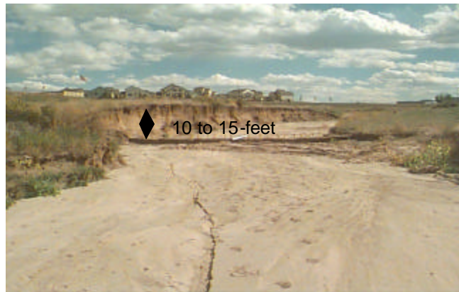
Figure 1. Channel degradation at Marcy Gulch.
