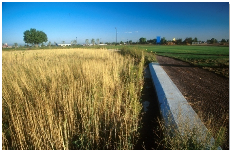
Photograph GB-2. This level spreader carries concentrated flows into a slotted pipe encased in concrete to distribute flows evenly to the grass buffer shown left in the photo. Photo courtesy of Bill Wenk.
