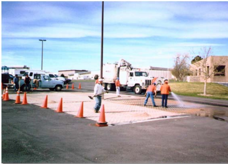
Photograph CGP-2. The Lakewood concrete grid pavement installation was one the first permeable pavement stormwater monitoring sites constructed by UDFCD. This photo was taken following construction in 1994.
