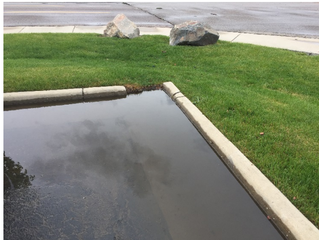
Photograph RR-3. Landscaping in the RPA (the grass swale) is too high to allow stormwater into the vegetation. Ensure a grade differential where UIA meets RPA. Photo courtesy of SEMSWA.
