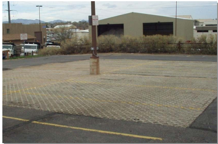
Photograph CGP-1. Concrete grid pavement installation in a parking area. The concrete segments along the perimeter of this installation showed wear that could have been mitigated with a concrete perimeter barrier.
