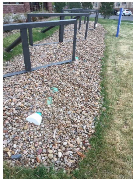
Photograph RR-2. A perforated pipe packed in gravel receives concentrated flow from the roof top of an office building and discharges the flow to a grass buffer. Photo courtesy SEMSWA.
