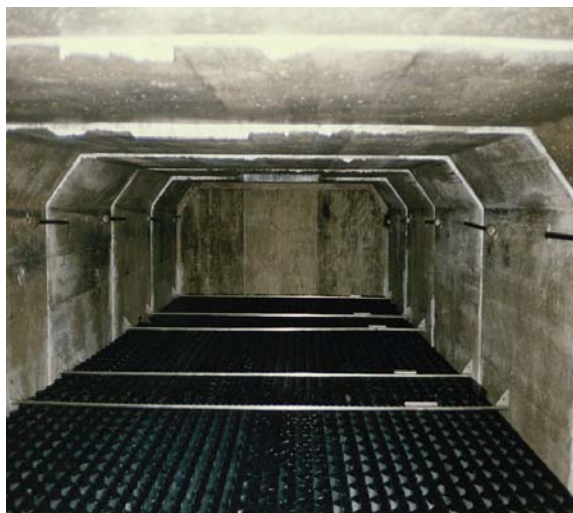
Photograph UG-2. Maintenance access to all chambers of an underground BMP is an important design consideration. Photo courtesy of Robert Pitt.
