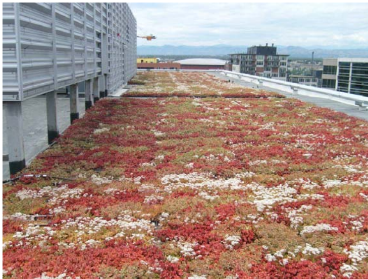
Photograph GR-1. EPA Region 8 building in downtown Denver. Photo courtesy of Weston Solutions.
