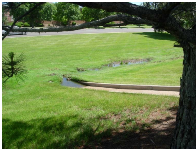
Photograph 6-2. A lack of sediment removal in this grass swale has resulted in a grade change due to growth over the deposition and ponding upstream.
