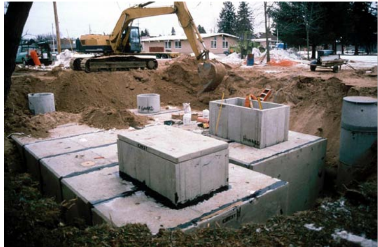
Photograph UG-1. Installation of an underground BMP (Photo courtesy of Robert Pitt).
