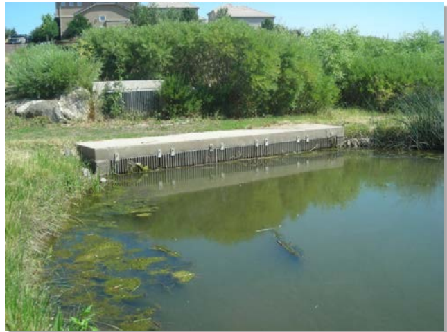
Photograph RP-2. This retention pond outlet structure is both accessible and functional while not interfering with the natural aesthetic.
