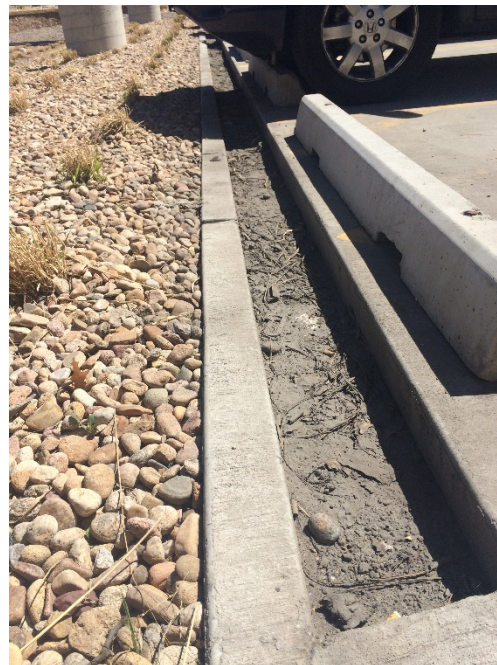
Photograph RR-2. This level spreader accepts and distributes concentrated flow while providing a place for sediment to be removed with a flat shovel. Note: When using this concept for quantifying volume reduction, use a grass RPA and create a free draining condition from the lowest flow point onto the RPA.
