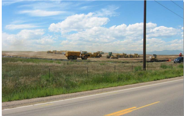
Photograph VB-1. A vegetated buffer is maintained between the area of active construction and the drainage swale. Photo courtesy of WWE.
