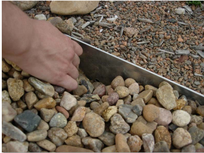
Photograph GR-2. The metal edge shown in Photo GR-2 has perforations near the bottom to allow flow into the drain.
