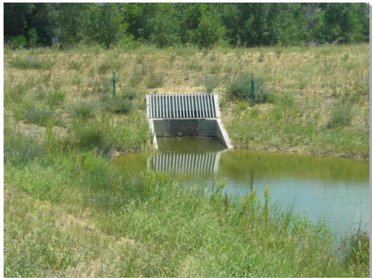
Photograph OS-1. Although each site is different, most sedimentation BMPs have similar outlet structures. Each structure should include a partially submerged orifice plate with a screen (or grate) protecting the orifice plate from clogging, and an overflow weir for flows exceeding the WQCV or excess urban runoff volume (EURV), when full spectrum detention is used.
