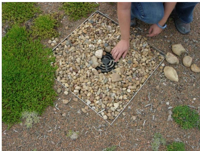
Photograph GR-3. Metal edging separates growing media from rock that surrounds the roof drain. It also serves to facilitate regular maintenance by limiting plant and root growth near the drain.
