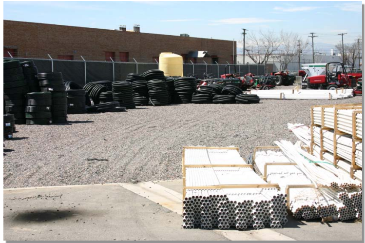
Photograph PG-1. This Denver installation of porous gravel provides volumetric treatment of the WQCV as well as a material storage area.
