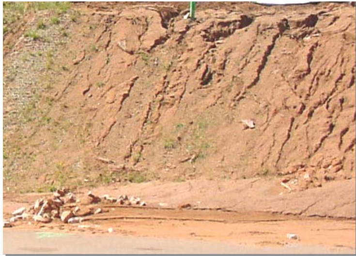
Photograph 7-2. Erosion is a common occurrence during construction activities, which can result in sediment movement off site and deposition in waterways when not properly managed. (Photo courtesy of Douglas County)
