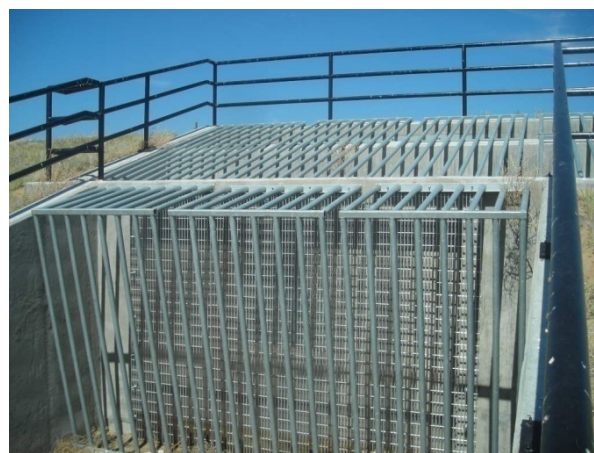
Photograph OS-5. Interruptions in the horizontal members of this trash rack and the spacing of the vertical members allow easier access to clean the water quality grate. A raking tool can be used to scrape the water quality trash rack.
