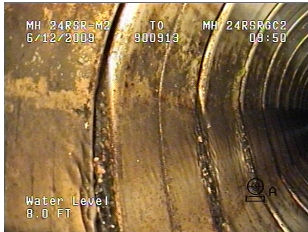
Sedimentation was not significant, but was noted at most pipe corrugations
