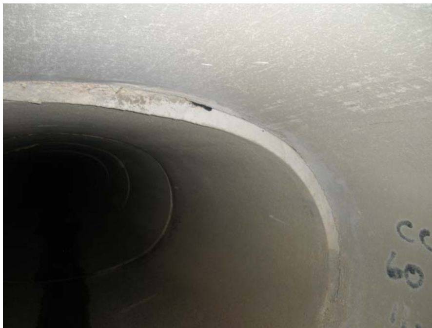
Photo 2 - Large offset in alignment near the top of the pipe
