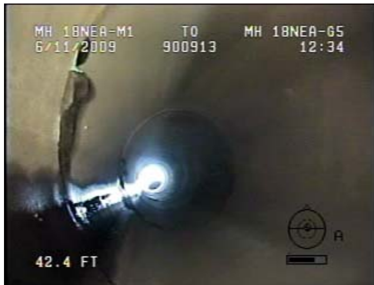
Pipe end was fractured during installation
