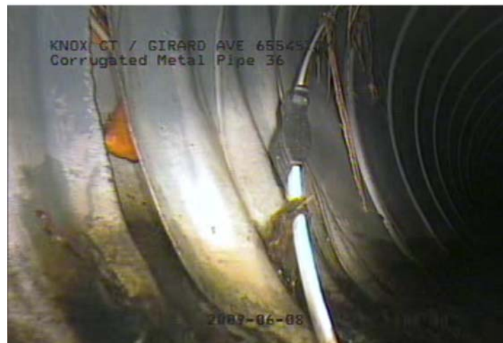
The pipe end was damaged during installation Part of the pipe end has broken and curled into the pipe and is obstructing flow
