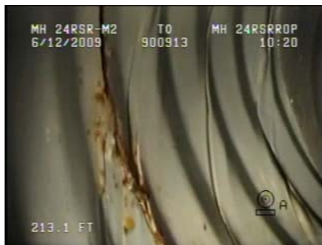
The sidewall of the pipe had a vertical tear Infiltration and moisture has heavily corroded the damaged
