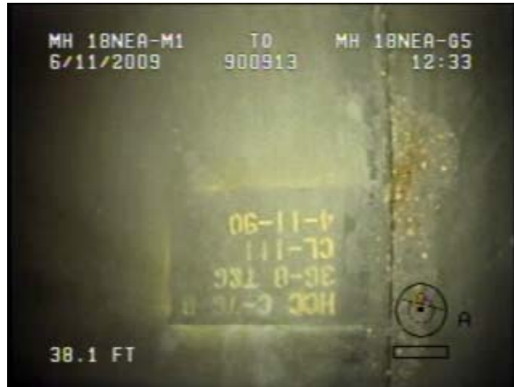
Surface abrasion noted along the crown of the pipe
