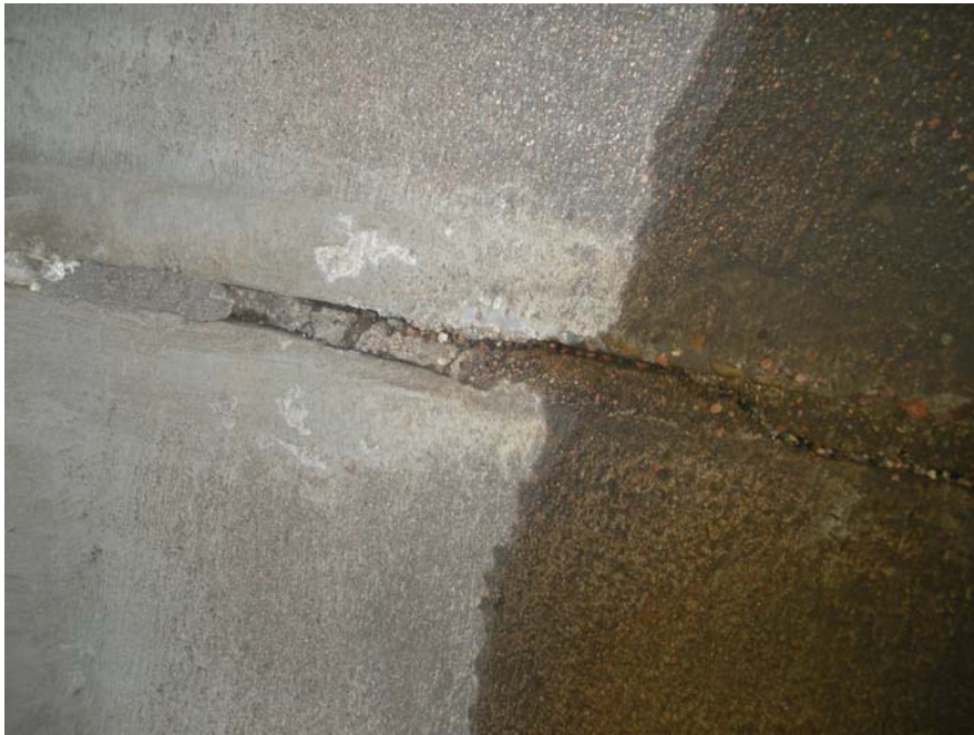
Photo 3 - Grout is failing near the invert of the pipe. Grout is completely washed away at the bottom of the pipe and sediment has filled the void
