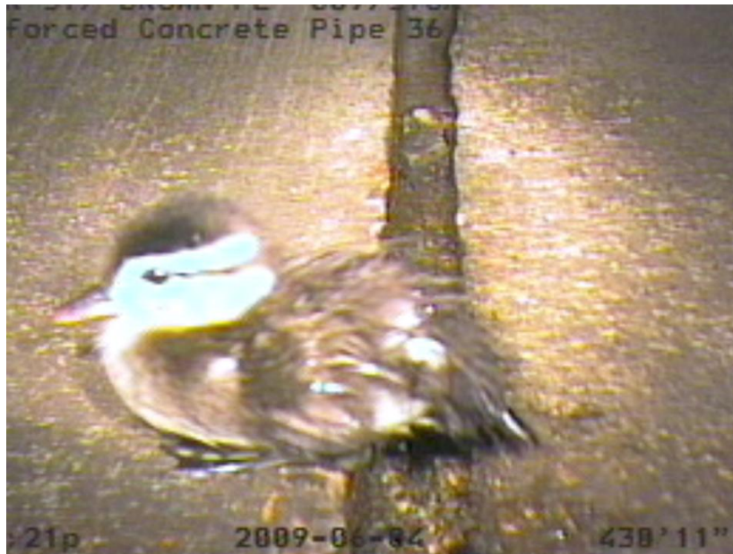
Slight joint separation as typical throughout (Note small bird shown for scale)
