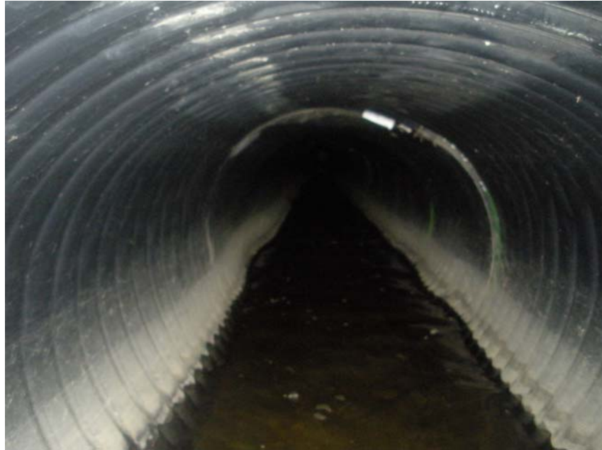
Photo 1 - The pipe is significantly out of round
