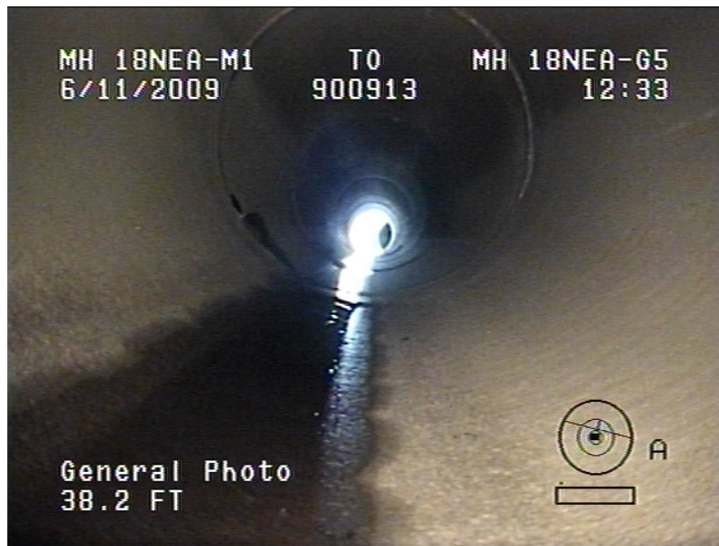
Pipe gasket exposed
