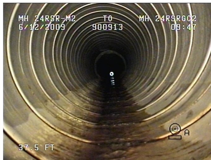
Medium corrosion was noted along the entire invert of the pipeline
