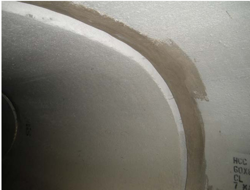
Photo 1 - Cement mortar patching near the upstream manhole. This patch is in excellent condition and fills an approximately 1" wide gap
