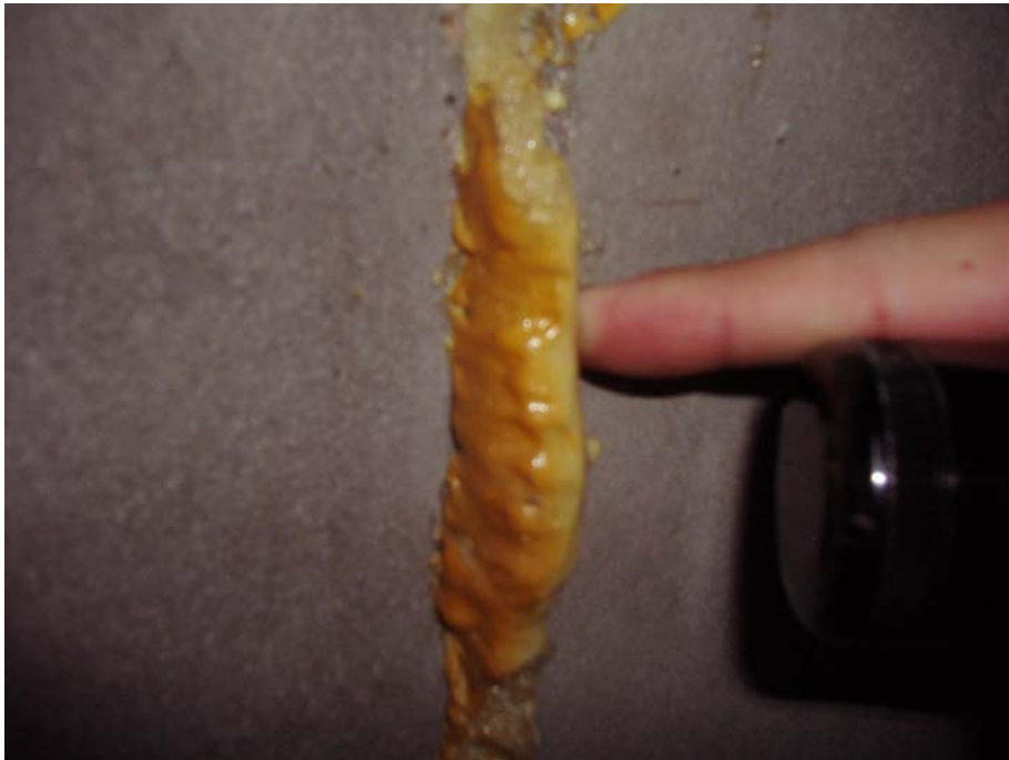
Photo 5 - The foam has expanded and penetrates up to ½” into the pipe
