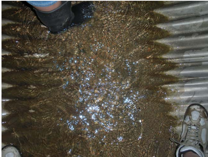
Photo 2 - Sedimentation at the bottom of the pipe has filled the corrugations with gravel and silt, typical for the entire pipeline
