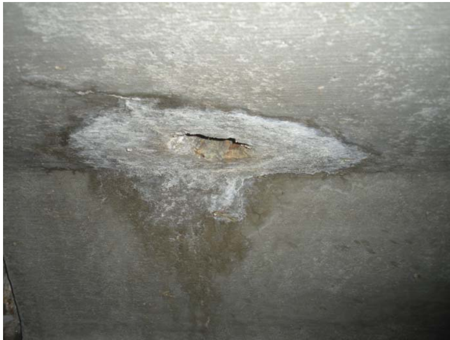
Photo 3 - The grout patch at this lifting hole has failed
