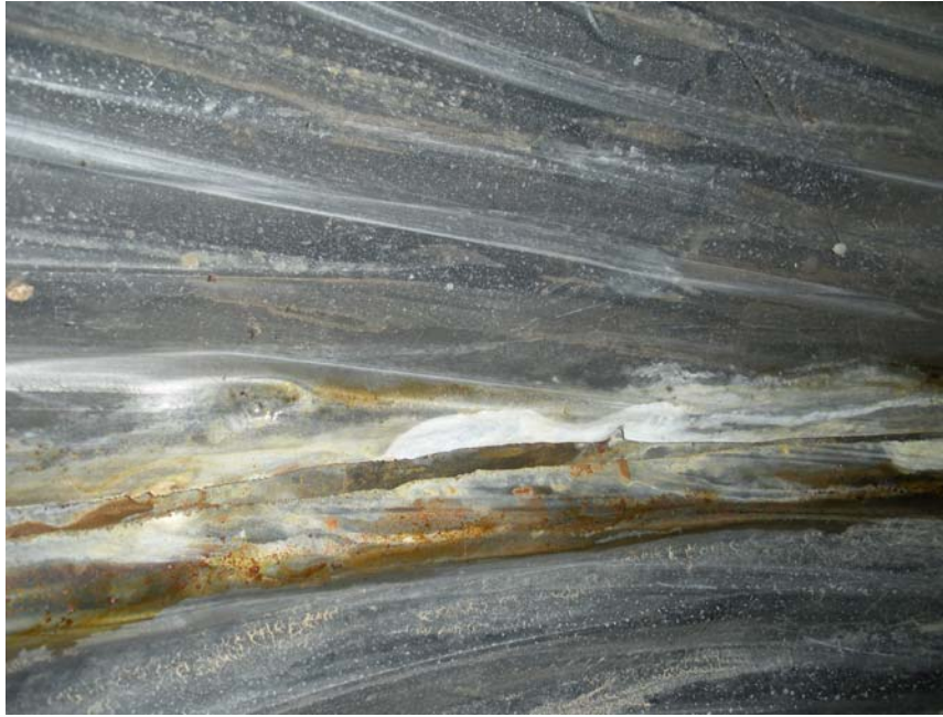
Photo 4 - Damaged joint – appears as if joint was damaged during construction
