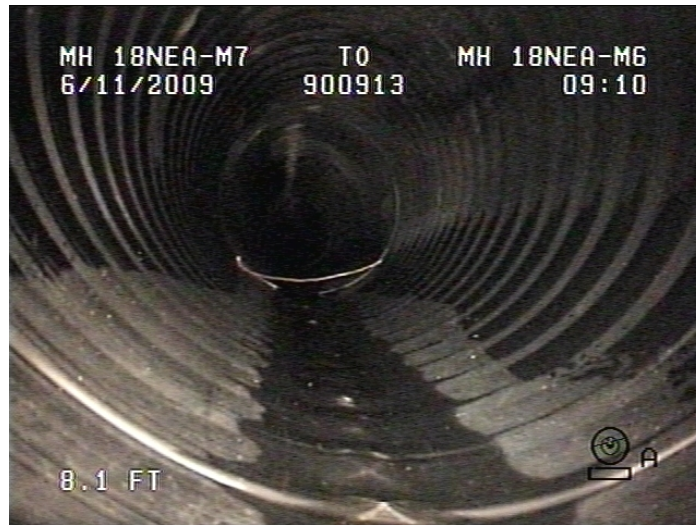
Pipe appears out of round (deformed)
