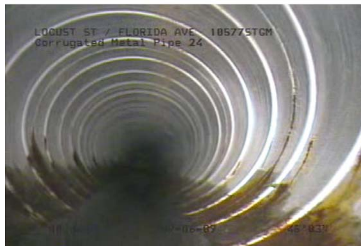
Medium corrosion was noted throughout the pipe – especially along the 2-3” above the base flow line
