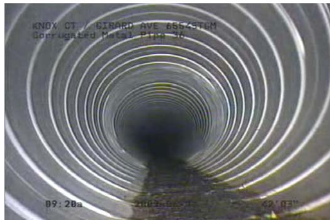
Light sedimentation was noticed throughout the inspected pipeline
