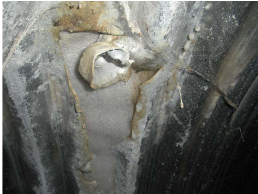
Photo 3 - Tear in the aluminum pipe wall likely experienced during installation. At this location, the pipe appeared to be wrapped with white foam, possibly in an attempt to patch the tear
