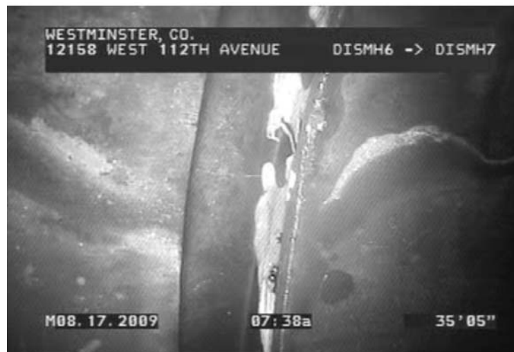
Pipe joint has separated by approximately 3-inches This separation does not seem to be obstructing the flow
