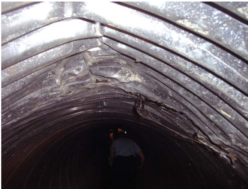
Photo 9 - Buckling along the crown of the pipe – damage likely caused during installation
