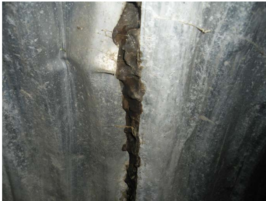
Photo 5 - Open separation at a damaged joint. The pipe is out of round and the bitumastic waterproofing is penetrating the opening.
