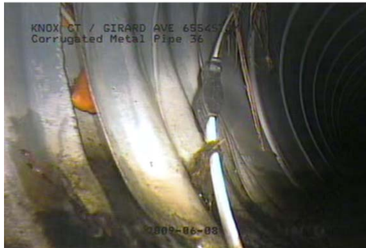
Pipe end is damaged and protruding into the flow Damage likely occurred during installation
