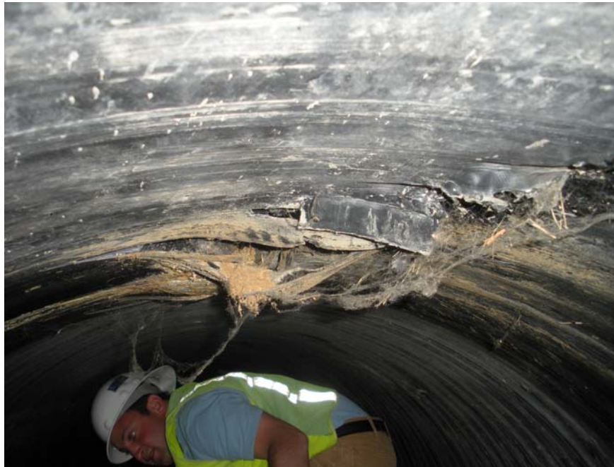
Photo 1 - Shear tearing of the inner layer of plastic observed at the top of the pipe
