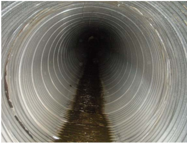
Photo 1 - Light corrosion at bottom of pipe
