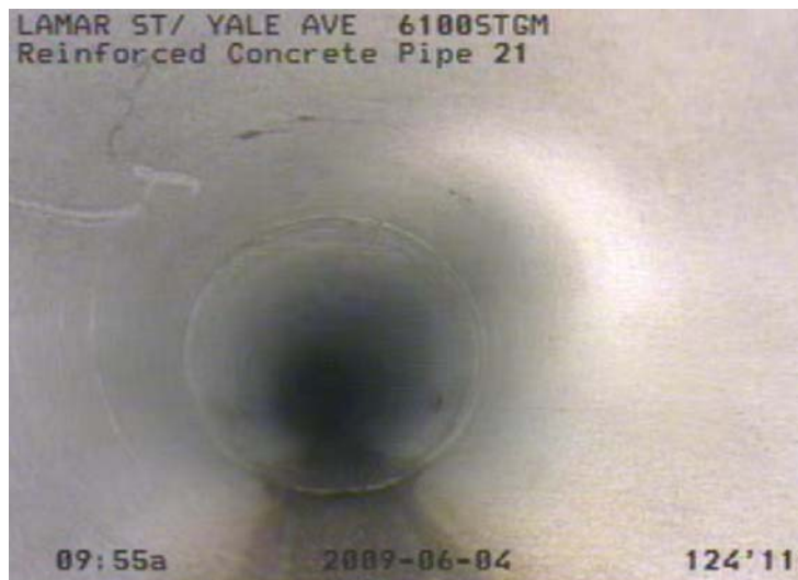
Light surface cracking along the crown of the pipe
