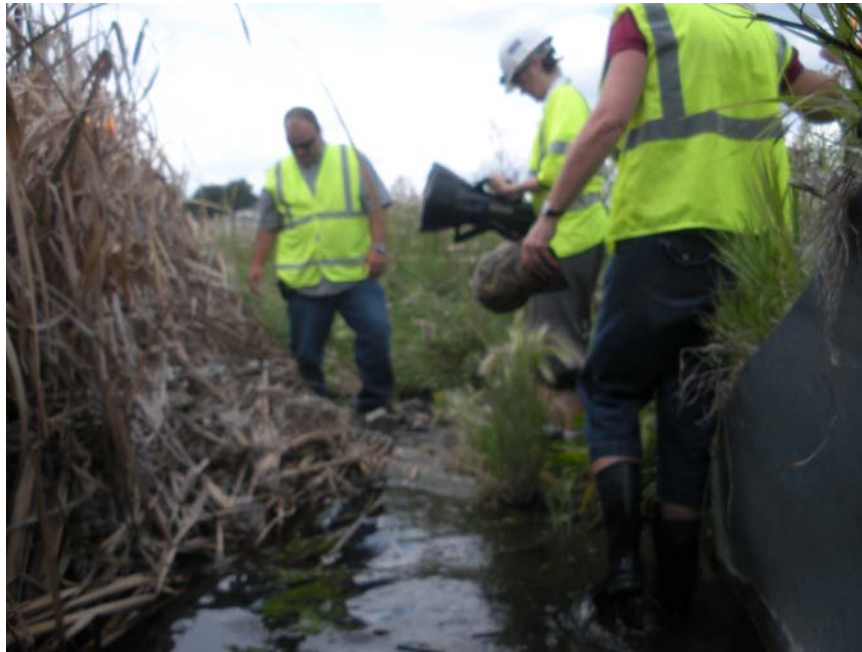
Photo 3 - A concrete energy dissipation structure installed at the pipe outlet invert is restricting drainage and creating permanent pooling within the pipeline
