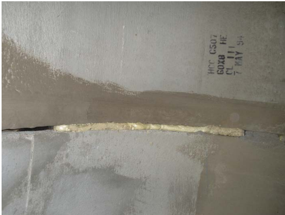
Photo 4 - Expanding foam at the top of the pipe. Notice the spots where it has failed
