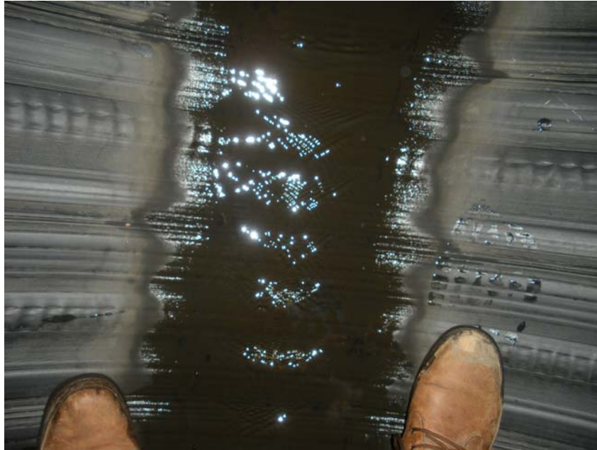
Photo 3 - The invert of the pipeline was free of any sedimentation or debris
