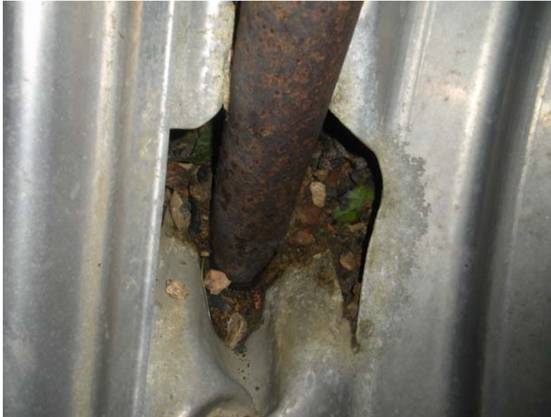
Photo 8 - Surface corrosion on damaged pipe wall. Note: 1/2" crushed rock bedding
