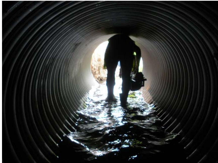
Photo 2 - The pipe is significantly out of round
