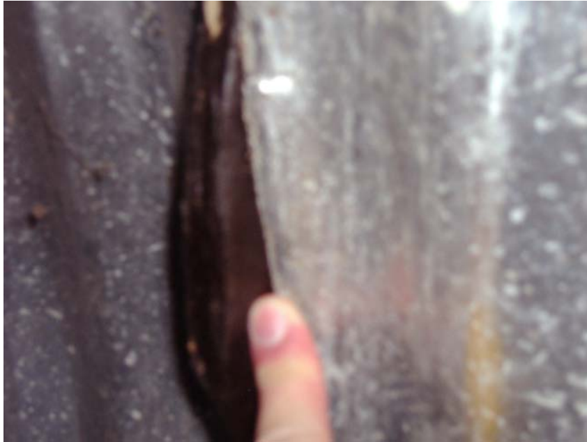
Photo 6 - Joint sealant material is squeezing into the joint
