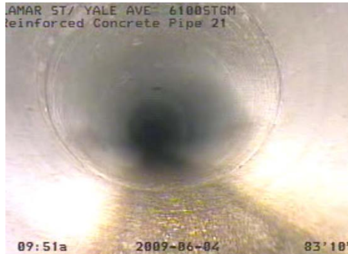
Light corrosion along invert of pipeline
