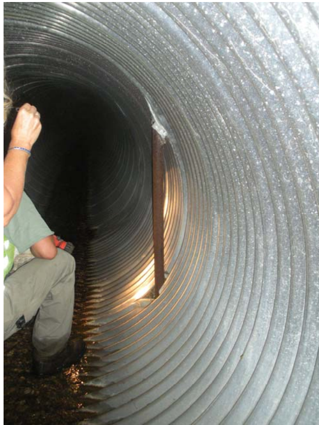
Photo 7 - Unknown utility installed thru pipe wall
