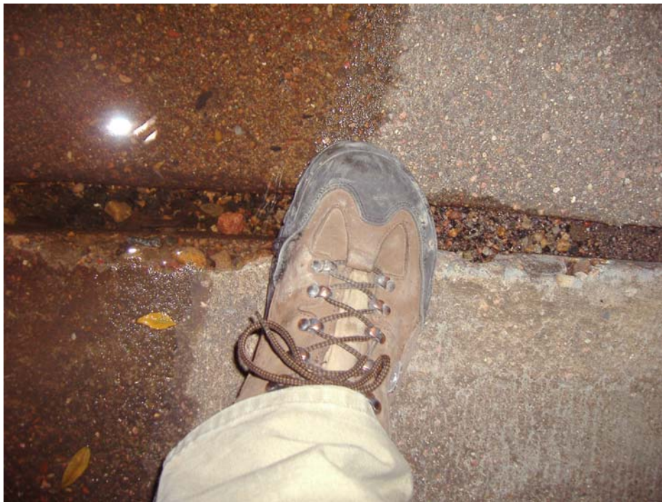
Photo 6 - Sediment has filled the void space at the joints at the invert
