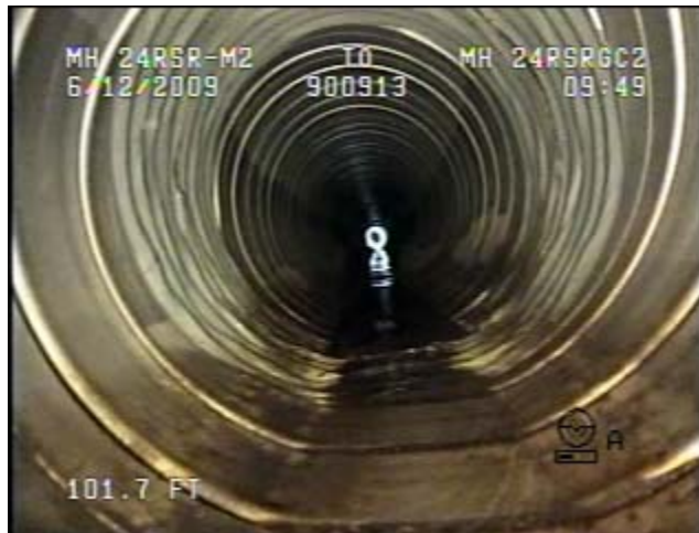
Medium corrosion was also noted at the corrugations of the pipe
