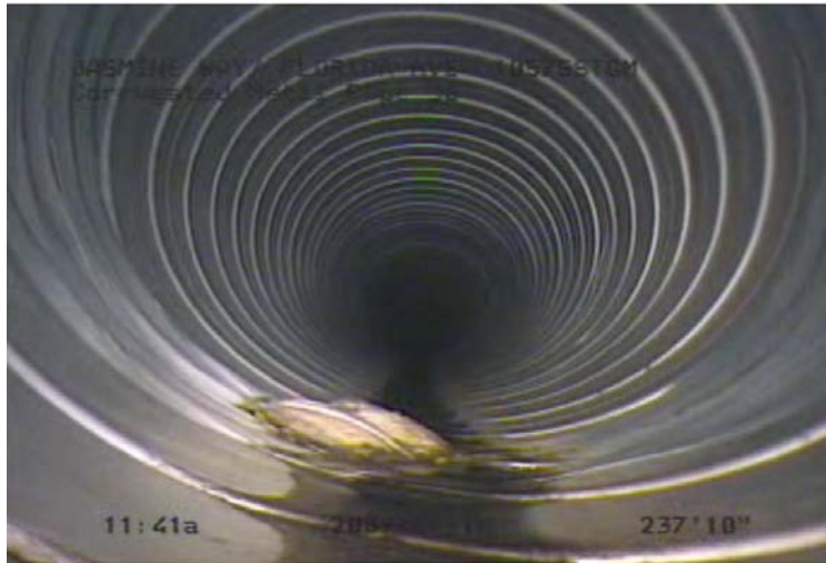
Pipe gasket material has rolled into the invert
