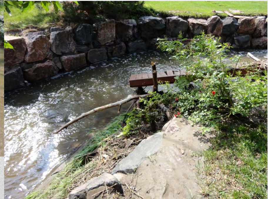
Tethered upstream wooden bridge was unseated
