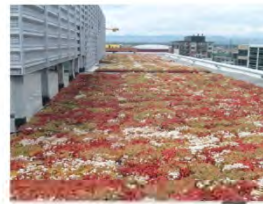
Photo GR-1. EPA Region 8 building in downtown Denver. Photo courtesy: Western Solutions.
