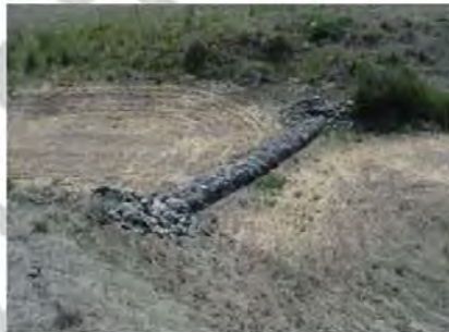
Photographs CD-1 and CD-2. Rock check dams in a roadside ditch and reinforced rock check dam in a small drainage swale. (Photo Sources: WWE; Douglas County)
