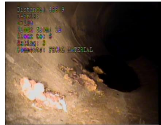
Fecal waste in a storm drain (Geosyntec Consultants)
