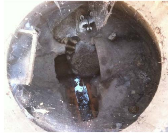
Raccoons in an urban storm drain manhole. Photo Courtesy: Andy Taylor, City of Boulder, CO.
