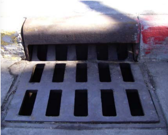
Retrofitted storm drain inlet, City of Boulder, CO
