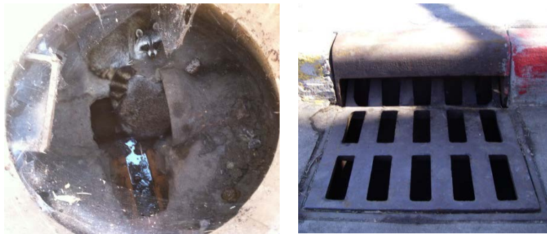
Raccoons inhabiting storm drain system (a) and retrofitted storm drain inlet (b). (Photos courtesy of Andy Taylor, City of Boulder, CO)
