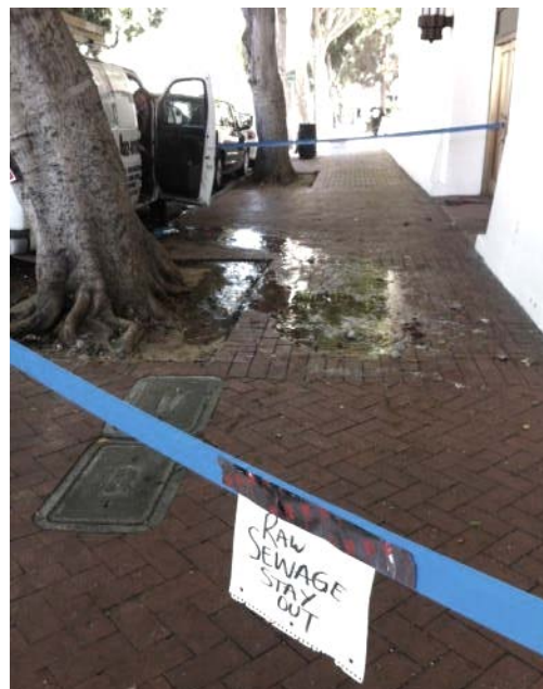
Sanitary sewer overflow. (Photo Courtesy Brandon Steets.)
