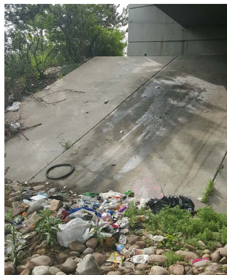
Homeless encampment beneath bridge with human excrement on concrete. (Photo courtesy of Darren Mollendor.)
