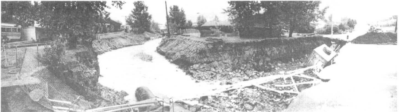
Composite photo taken on August 5 looking downstream at Massey Draw from Carr Street in Jefferson County. Road maintenance crews helped direct water toward the main channel during the storm by constructing a temporary earth dike shown in photo.
