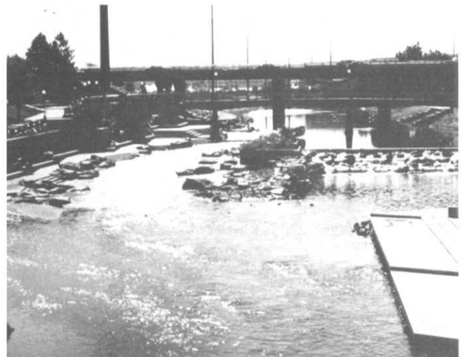
Looking directly upstream, the existing plaza is in the lower right with the new diversion dam center right and the new boat chute and plaza center left.
