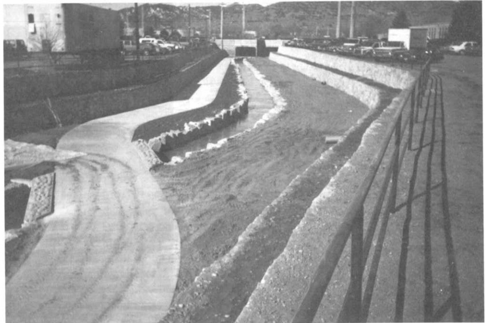
Goose Creek, looking upstream toward 30th Street in Boulder, prior to revegetation.
