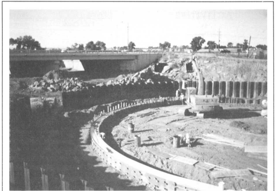
Construction of a two-tiered, 12 foot high, sheet pile and rock drop structure on Sand Creek downstream from Colfax Ave. The drop structure is part of a $1.1 million project sponsored by Aurora and the District.
