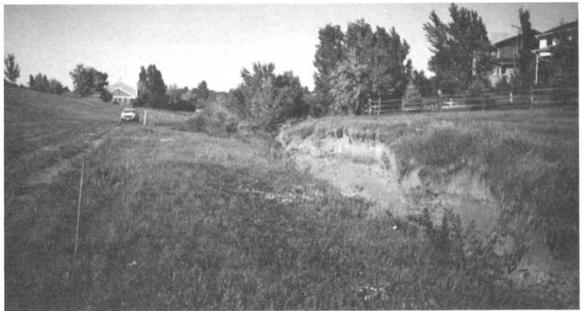
Degradation of the low flow channel was causing formation of tall vertical banks which caused a safety hazard.
