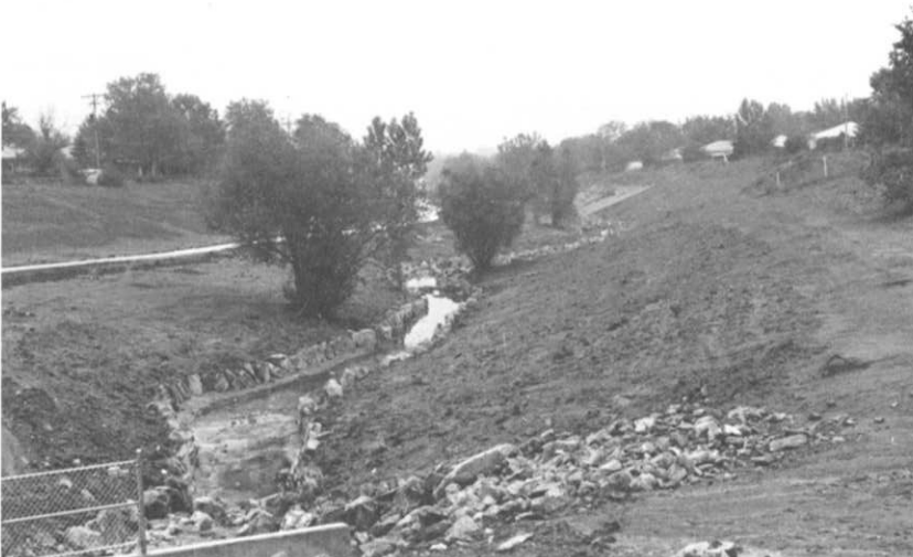
Right After: The project was completed in early 1991. The banks were laid back and a boulder lining was installed along the low flow channel.
