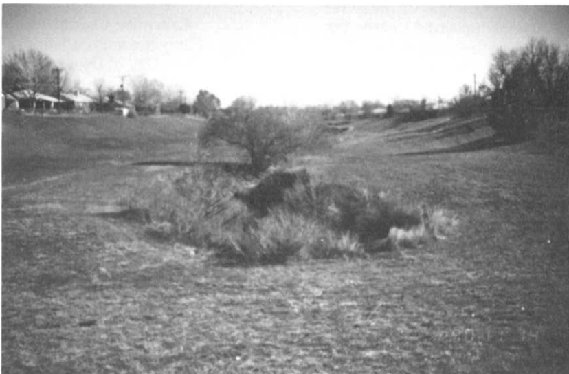
Before: Degradation of the low flow channel was causing vertical banks.
