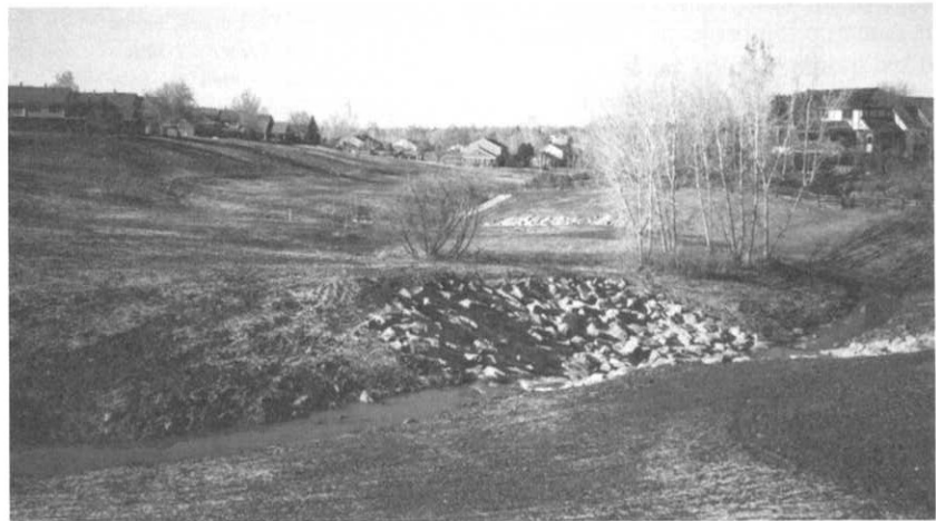
The rehabilitation project consisted of installation of grade control structures and laying back the vertical banks. Notice how the project protected many of the existing trees near the low flow channel.
