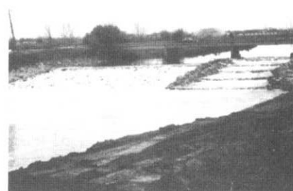
The drop structure consists of a grouted boulder section at a 10:1 slope (left) and a boat chute (right).
