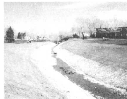
Interlocking cellular concrete block erosion protection was installed in West Harvard Gulch under the direction of project engineer Frank Rosso. Once vegetation is established it will be difficult to see the concrete.
