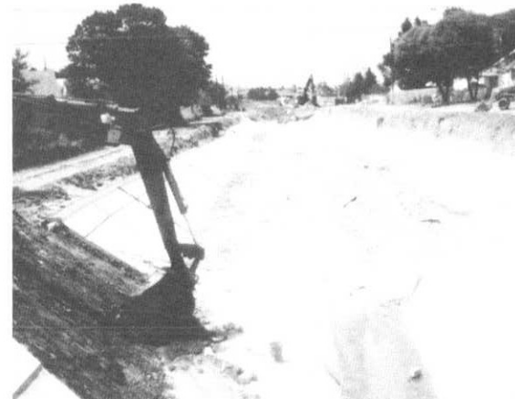
Little Dry Creek construction in Westminster. Limited right-of-way forced a concrete lined channel in order to provide 100-year flood protection.
