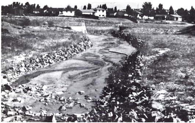
Native grass-lined channel with riprap lined low flow channel in sandy soil. This is Meadowwood Channel in Aurora.
