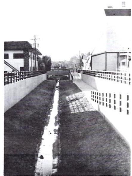
Recently dedicated Little's Creek channel in Littleton. Channel consists of concrete walls, grass bottom, trickle channel and maintenance trail.
