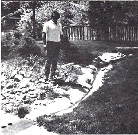
Figure 5—Paved rundown to trickle channel.
