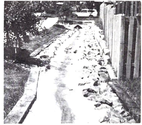
Figure 9—Concrete trickle channel in an Arapahoe County subdivision.
