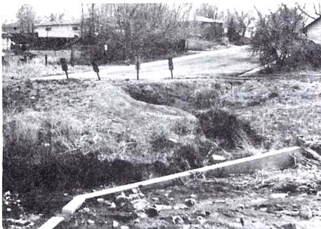
Figure 12—Lack of a runoff to the channel invert on Sanderson Gulch in Denver.
