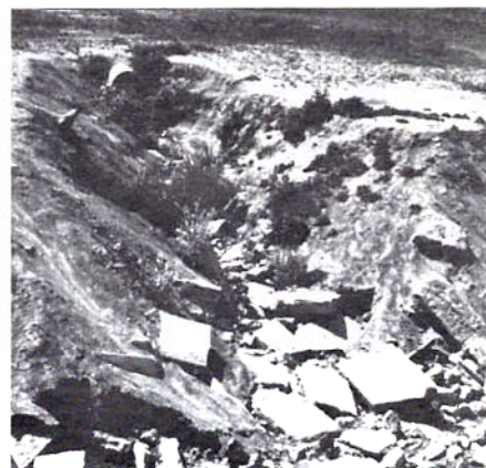
Figure 4—Erosion at storm sewer outlet.
