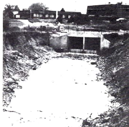
Figure 2—Erosion and degradation on Bear Creek in Boulder.
