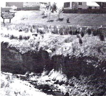
Figure 3—Degradation on Little Dry Creek in Arapahoe County.
