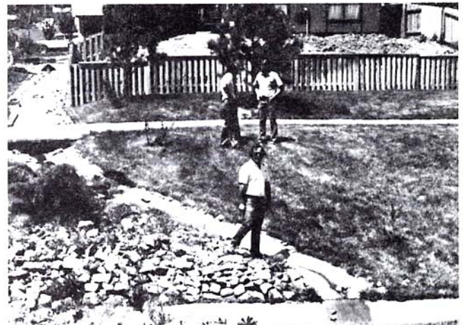
Figure 13—Concrete runoff to the trickle channel.
