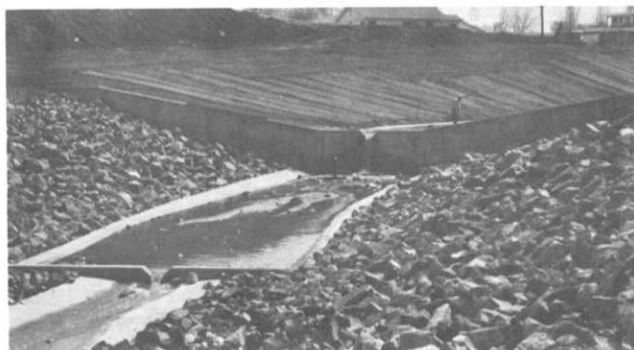
The District is trying a concrete drop structure to try to get away from the vandalism problems with gabion structures. The rip-rap will be buried and seeded, thus leaving only the concrete wall in sight.
