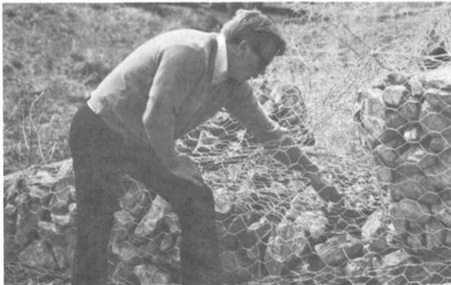
Vandalism of gabion structures continues to be a serious maintenance problem.
