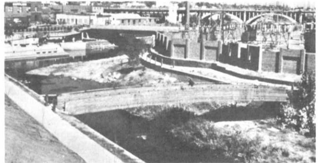
Figure 1.—Centennial Bridge. The left abutment connections will shear under pressure from high water or debris and the bridge will swing to the right bank.
