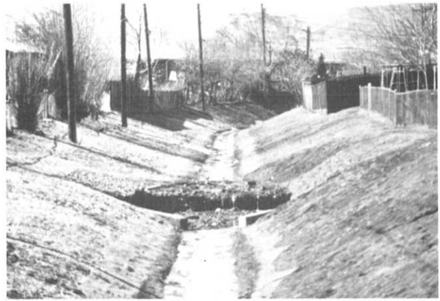
Improvements on one reach of North Sanderson Gulch consist of a grass lined channel, concrete low flow channel and gabion drop structures.
