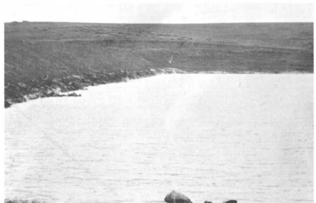
Englewood dam during the May 1973 flood. A new emergency spillway is being constructed to meet requirements of the State Engineer.
