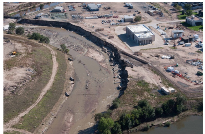
Flood waters on Sand Creek at the confluence with the South Platte River eroded approximately 100 feet of the outside bend into the Metro Wastewater Reclamation plant property, leaving a 25 foot vertical bank.
