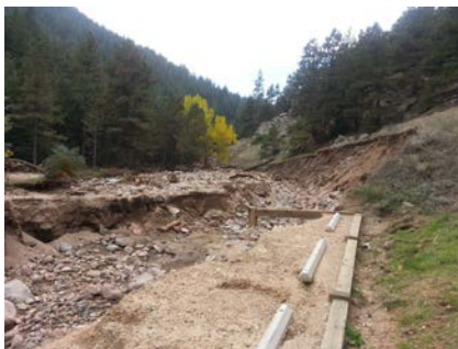
New channel cut by Fourmile Canyon Creek in Boulder County near UDFCD border. Actual creek channel is left of photo. Damaged parking area served the Anne U. White Trailhead prior to the flood.
