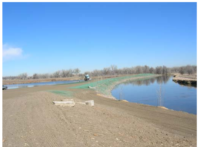
Before and After (prior to revegetation) of West Bank at Adams County South Platte Fishing Lakes
