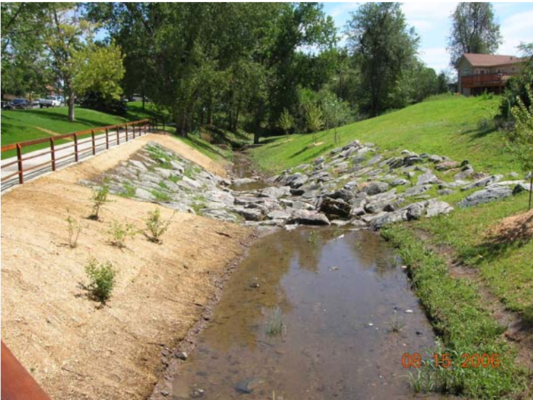
West Harvard Gulch in Denver east of Clay Street. In this mature neighborhood there was little option to this linear alignment. The drop structure will control the grade of the stream and prevent the channel from again becoming incised.
