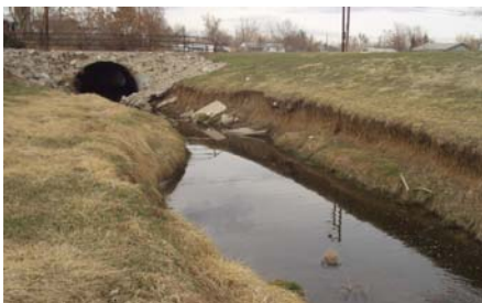
Incised channel upstream of Florida Avenue
