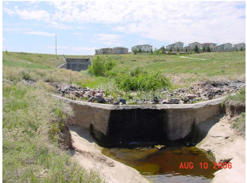
Grade control structure located downstream of the Wildcat Reserve Parkway crossing culvert and impact basin. The degradation at structure face is 7 feet with another 3 feet in the plunge pool.
