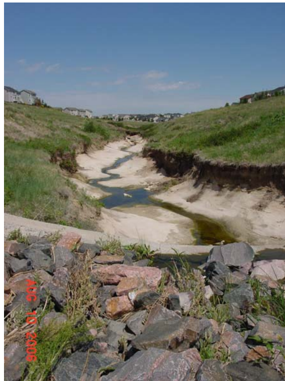
Looking downstream over the grade control structure. Notice the severe erosion, 4 to 6 feet into bedrock.
