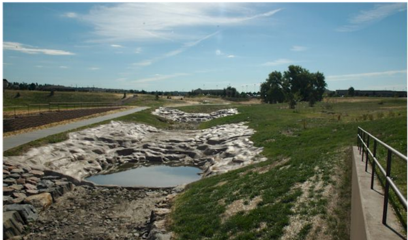
View of the completed project looking upstream from Twenty Mile Road. The large drop structure is in the immediate foreground. The extended approach section is for underground utility protection. The mature cottonwood trees identify the preserved oxbow location.
