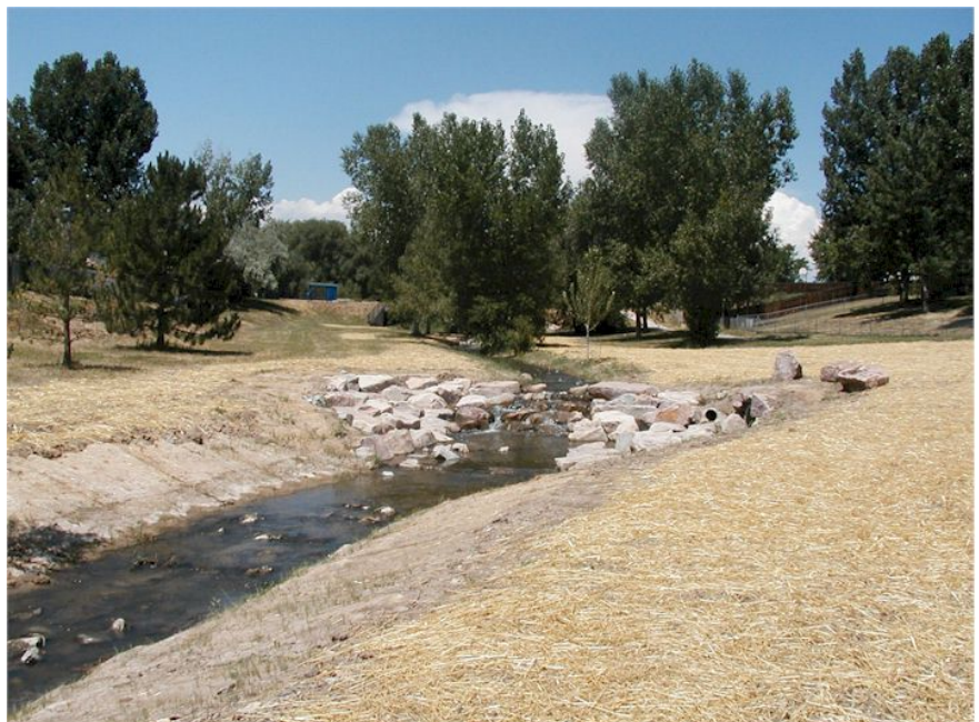
Little Dry Creek north of 80 th Avenue in Arvada. This grouted boulder drop structure has stabilized the channel within the park and protects a sanitary sewer line that had been completely exposed by erosion.
