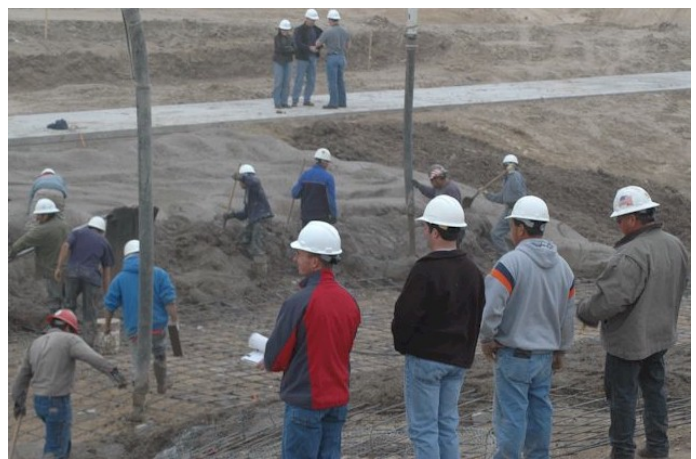
Matt Erichsen with Kiowa Engineering Corporation and Chris Castelli with Farnsworth Group (center foreground) provided interactive construction observation. The final surface treatment cannot be completely conveyed through design drawings, rather through skilled field control and a willing contractor.
