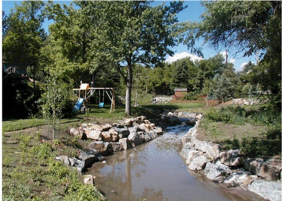
Lena Gulch in Lakewood between 20 th Avenue and Youngfield Street. Boulder edge channel built within a confined backyard drainageway easement
