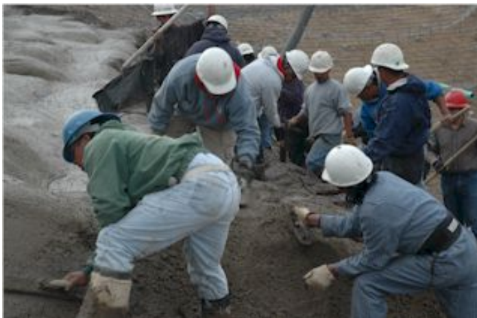
Concrete placement on April 8, 2005, for the largest of the sculpted concrete drops started at 7:00 am and was completed in the late afternoon. The entire workforce of Naranjo Civil Constructors was involved. This brings new meaning to the term, teamwork.
