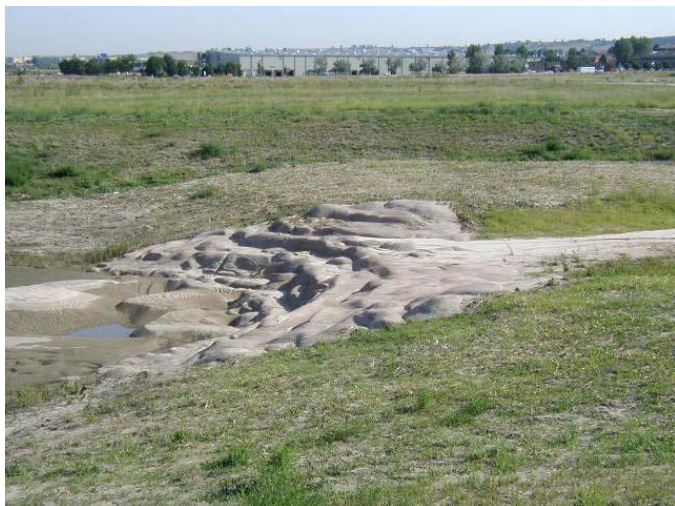
Long's Way Tributary sculpted concrete drop structure.
