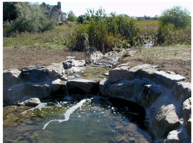
Greenwood Gulch drop structure. The sheet pile cutoff wall is hidden behind the grouted boulder drop structure.
