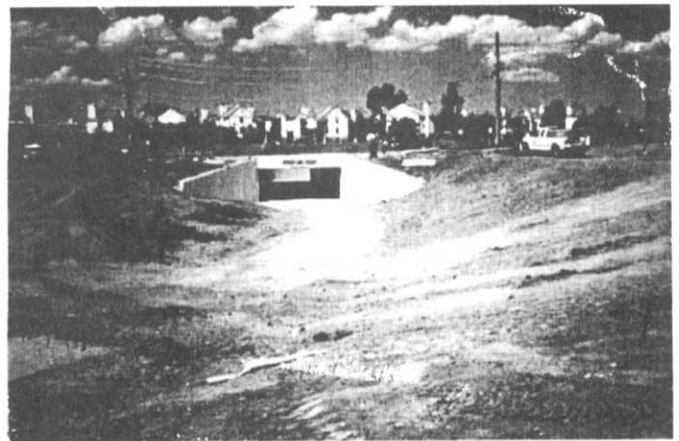
A bike path crossing structure under Sheridan Blvd. in Westminster provides additional flood carrying capacity for Little Dry Creek.
