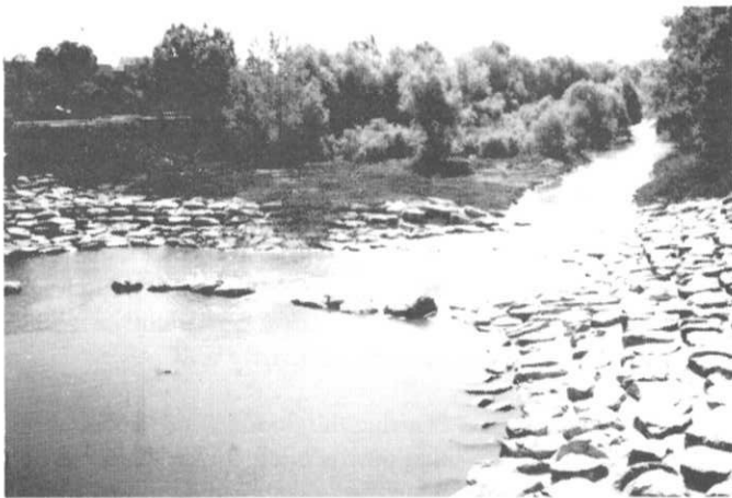
A grouted sloping boulder drop structure on Cherry Creek upstream from Cherry Street in Glendale.
