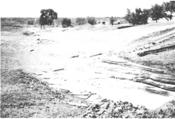
Grade control structures were built to resemble natural rock outcroppings at Grange Hall Creek in Northglenn.
