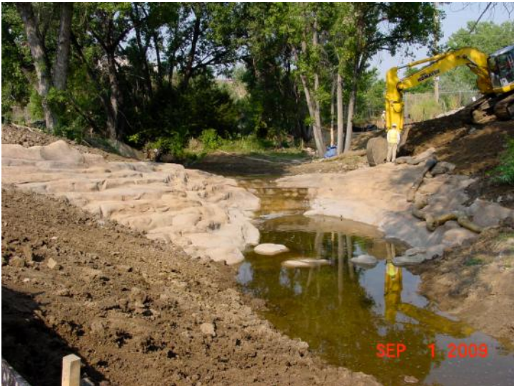
McIntyre Gulch sculpted concrete drop structure at the confluence of the North and South Branches.
