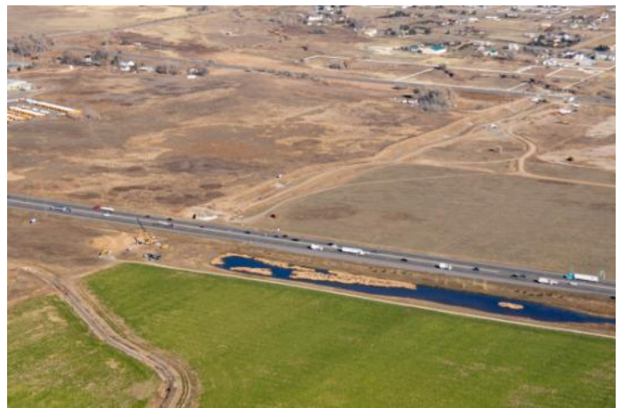
McKay Lake Drainageway, phase one channel construction nearing completion between I-25 in the foreground and Washington Street in the background.
