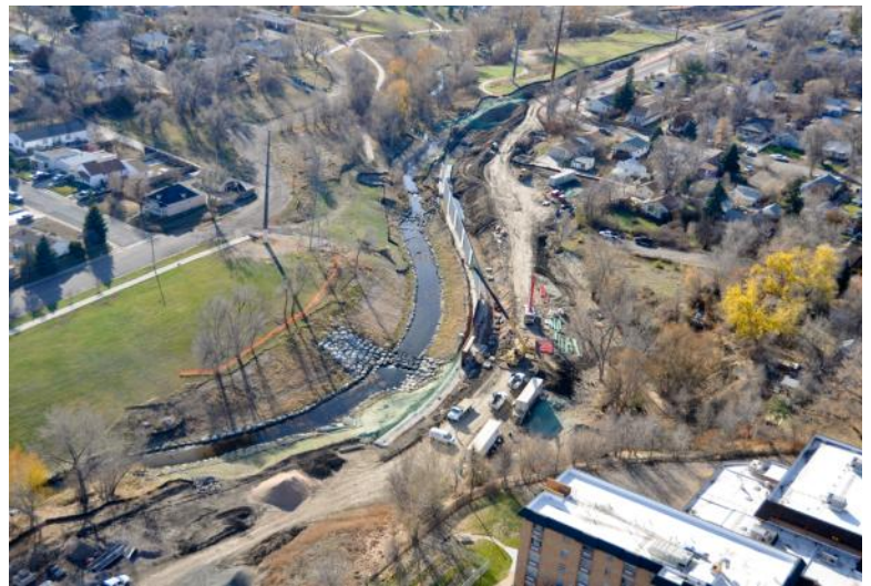
Drop Structure No. 2 on Lakewood Gulch west of Knox Court in the "Oxbow Area"
