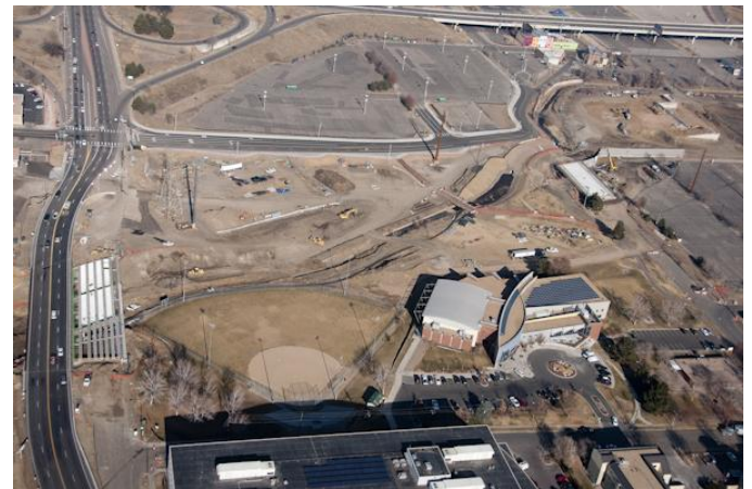
Lakewood Gulch work is progressing. This photo was taken on December 22, 2010 and includes the Federal Boulevard and Decatur bridges as well as the RTD light rail bridge. View is looking north.
