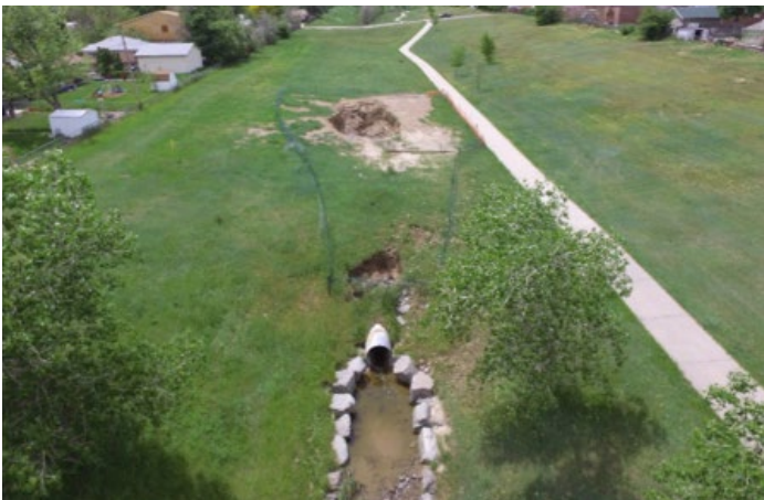
Pre-Construction Aerial of sinkhole
