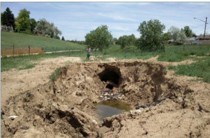
Pre-Construction View of sinkhole
