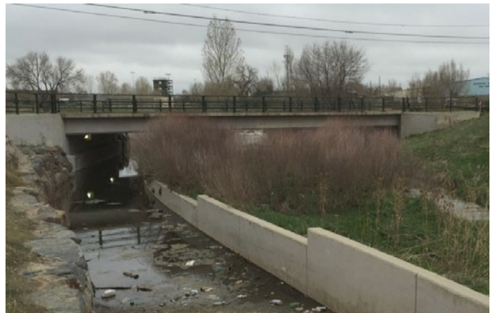
Pre-Project at Lowell Underpass – note the continually flooded underpass
