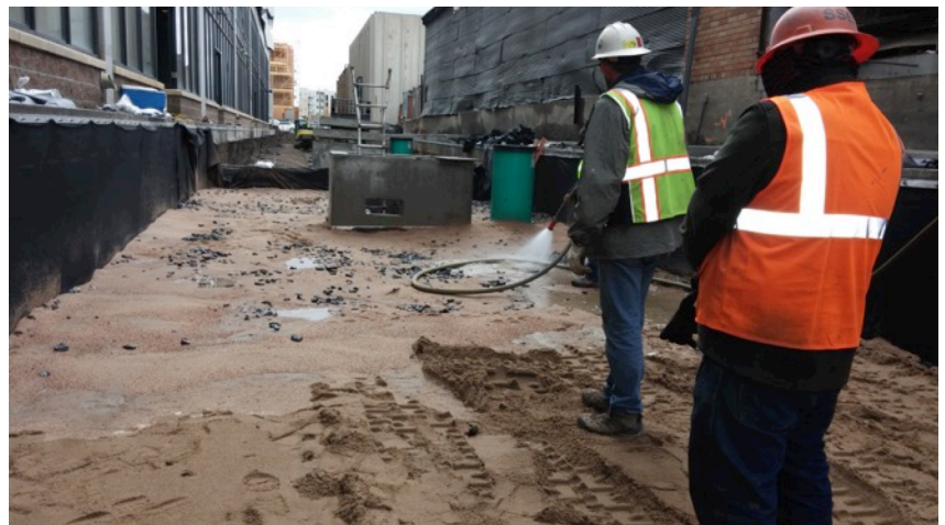
A crew at Industry washes filter media into the structural base of this permeable pavement section. In the distance a second section will be constructed without filter media. Both sections will be monitored for water quality.
