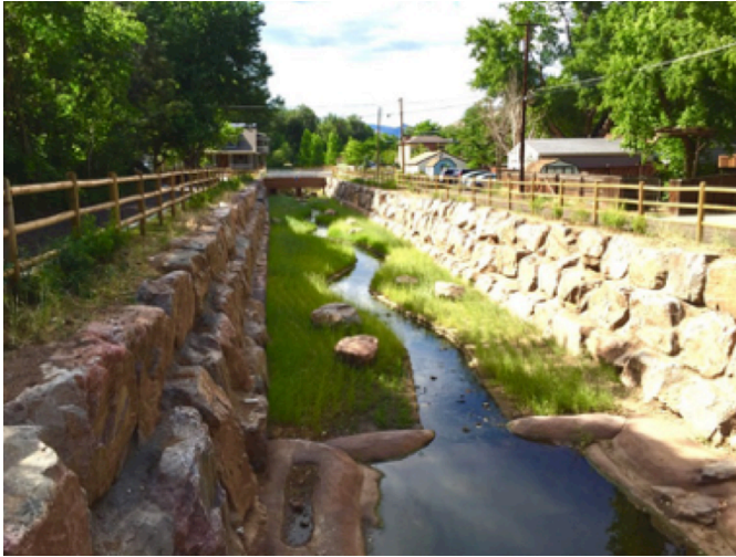
Alleyway Boulder Wall Channel on West Fork of Kenney's Run - Envirolok® bags on bottom
