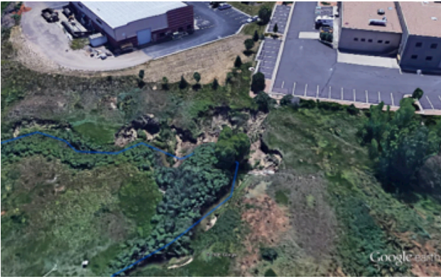
Stream bank erosion at location two.
