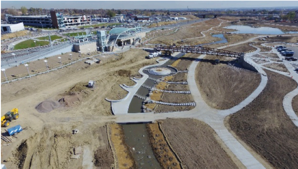
View of nearly completed Little Dry Creek, looking east toward Federal Boulevard. The Westminster Station is on the Left.
