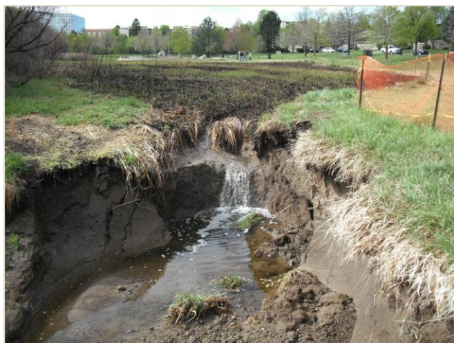
Looking south at the existing channel, erosion threatens community of wetlands and overall corridor.
