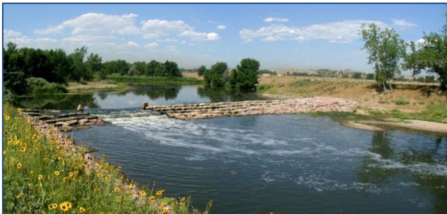
This re-aeration structure is a product of UDFCD's capital improvement program, matching local funds to construct infrastructure that manages river flows safely and improves water quality in the process.
