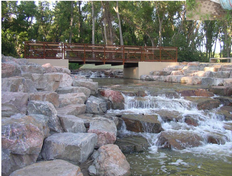
Finished drop structure looking upstream at Marcy Gulch. (Inset) Trout caught in Marcy Gulch
