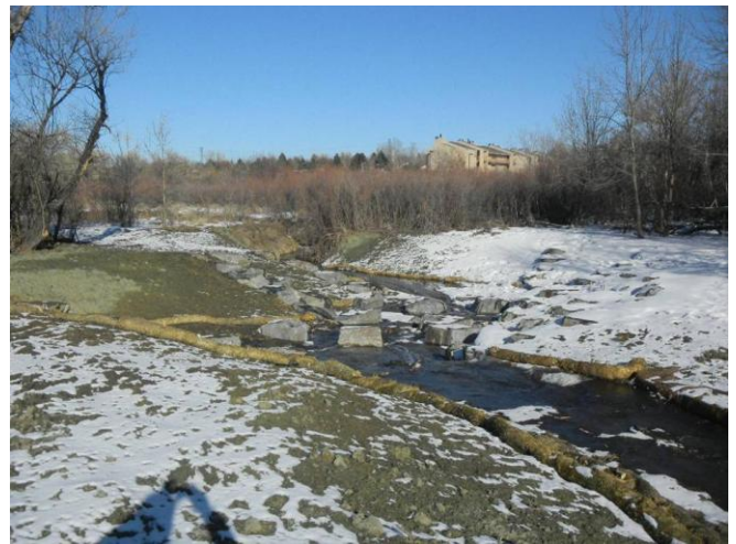
Looking north at improved corridor, partially grouted drop structure stabilizes the channel and protects upstream wetlands
