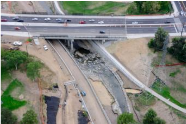
Lakewood Gulch drop at Federal Boulevard. Photo date is September 12, 2011. This was the largest of the six drop structures built as a part of the RTD West Corridor FasTracks Project. View is looking east and downstream.
