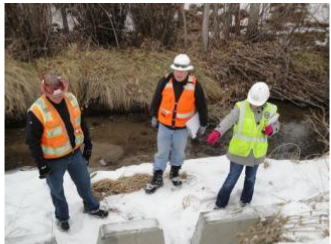
Joanna is seen here conducting a punch list walkthrough on December 12, 2011. This was the last in a series of RTD West Corridor substantial completion inspections for various drainage elements. Also in the photo are Ryan Espoy (left) and Barry McClung (center) with DTCC.
