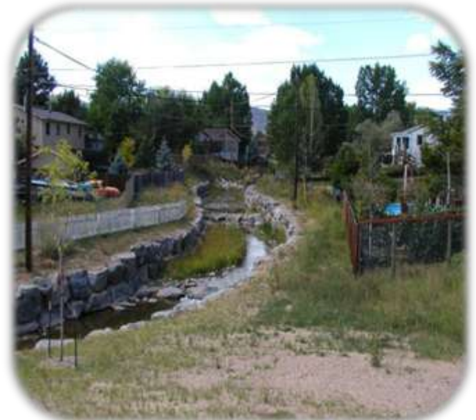
This view of Massey Draw shows the tight corridor in which the boulder walls and drop structures were built
