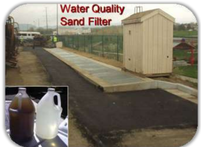
New open-bed sand filter test site. This BMP may offer an economical solution for ultra-urban stormwater quality treatment
