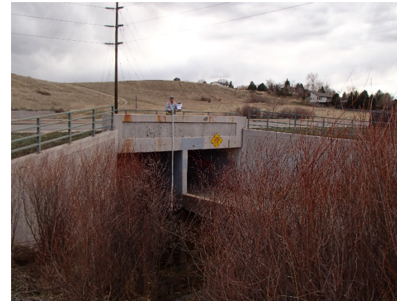
Reach WC-4: Structure 31 – Simms Street (1) 12-ft by 10-ft RCBC (1) 12-ft by 9-ft RCBC
