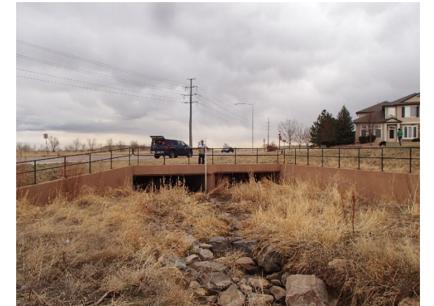
Reach WC-3: Structure 32 – West Quincy Avenue (1) 16-ft by 7-ft RCBC with 2 feet filled in (1) 16-ft by 7.5-ft RCBC with 2.5 feet filled in
