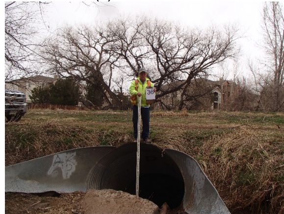
Reach WC-2: Structure 36 – Warrior Canal and Maintenance Road (1) 96-inch by 60-inch Elliptical CMP
