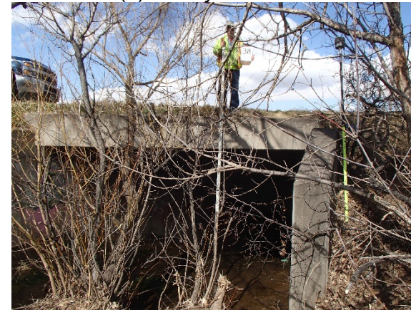
Reach WC-1: Structure 38 – Hampden Avenue/Highway 285 (1) 15.5-ft by 6-ft RCBC (Modified Drop Inlet) (7-ft by 6-ft RCBC at Throat)
