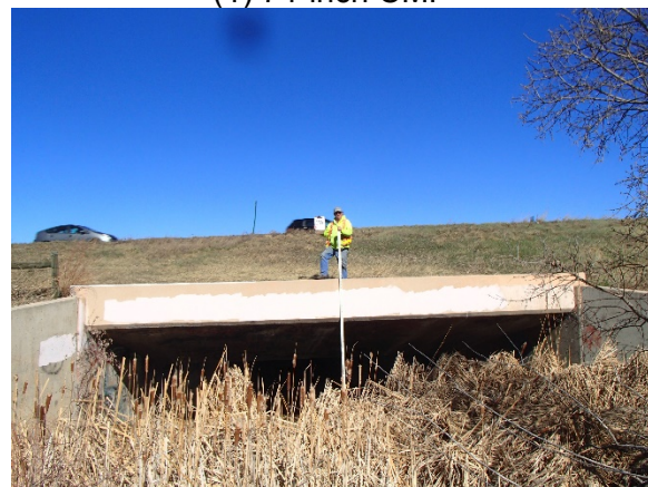
Reach WC-4: Structure 25 – C-470 (1) 35-ft by 6-ft RCBC (Modified Drop Inlet) (16-ft by 6-ft RCBC at Throat)
