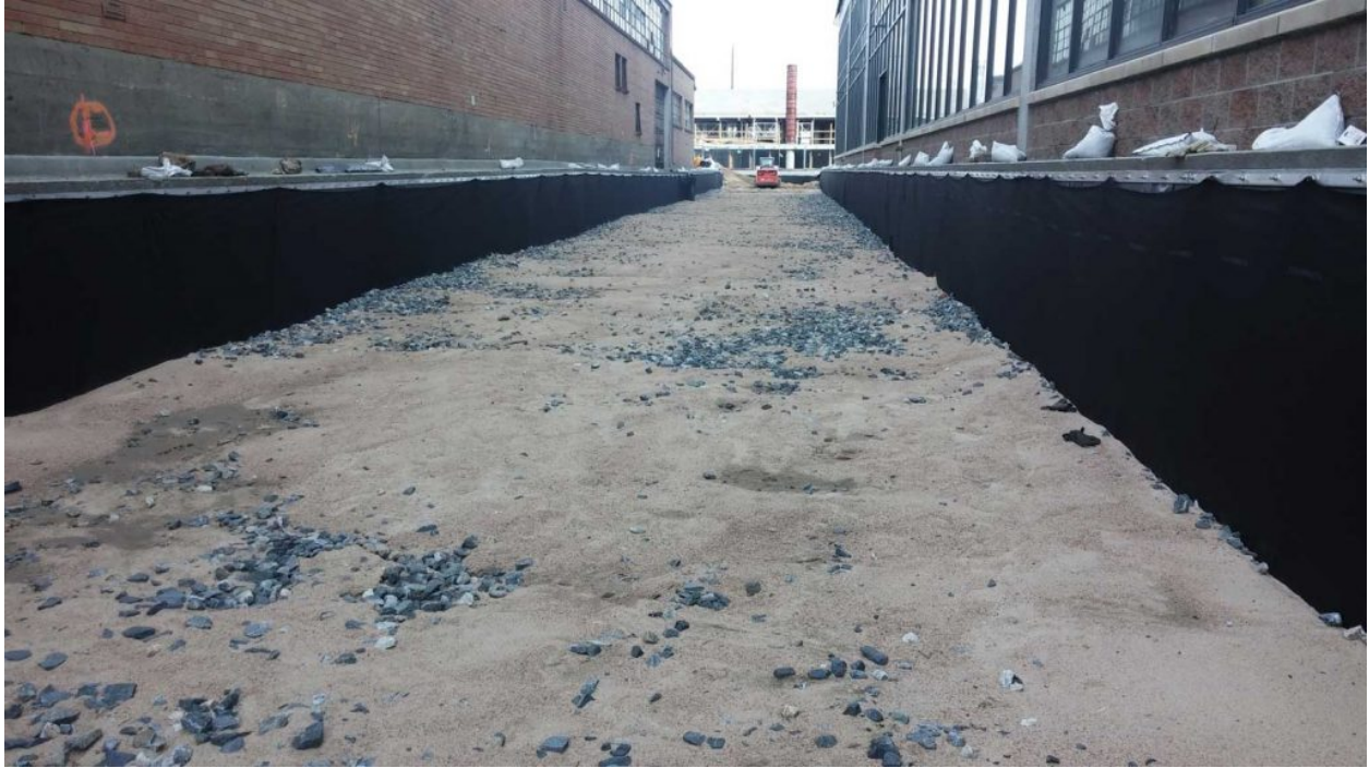
The filter layer in Section 2 was constructed by placing the No. 2 aggregate first and washing in CDOT Class C filter material
