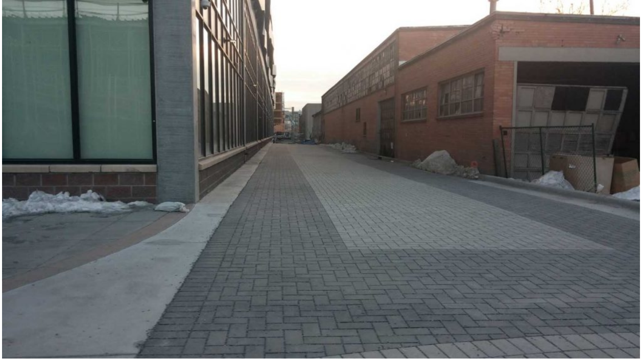
Openings between the bricks are filled with small (No. 89) aggregate. This photo shows Section 1 complete.
