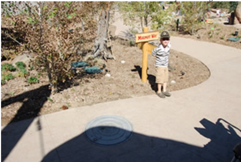
Stormsewer Sampling Manhole
