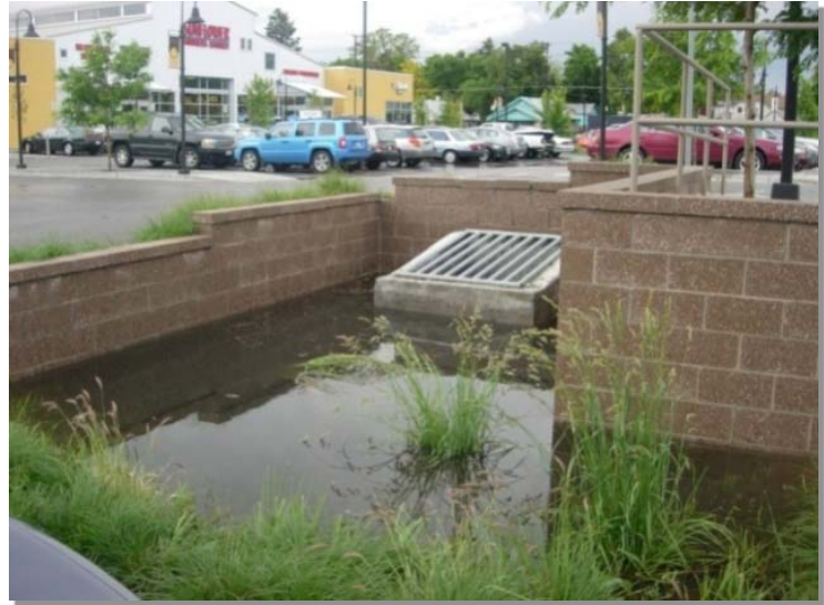
Photograph EDB-3. Although walls may complicate maintenance access, this outlet structure is relatively hidden from public view. This photo was taken shortly following a storm event.
