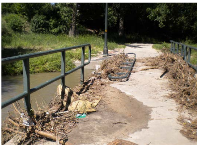
Photograph 10-5. Most of the “break-away” rails on this crossing failed to break despite the capacity lost to debris.
