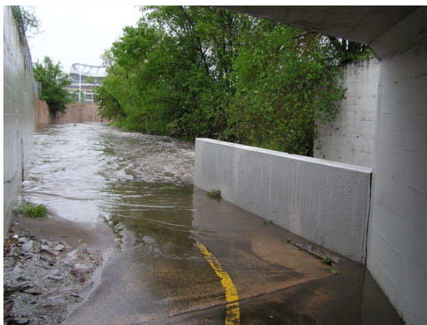
Photograph 10-1. Frequently inundated channels pose a high threat to public safety, especially in a walled channel where water can rise rapidly and egress is limited.
