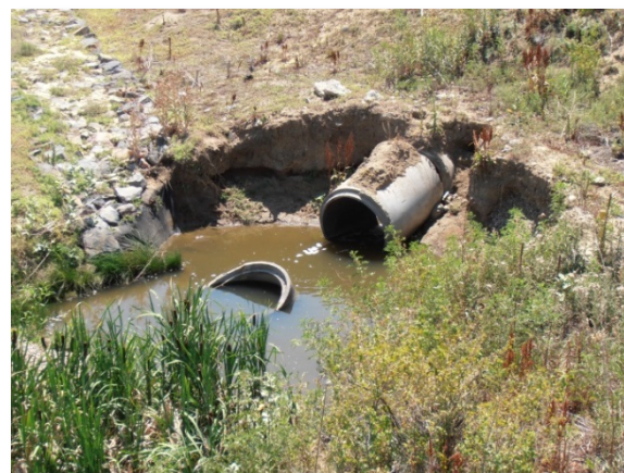
Photograph 9-29. Pipe end failure resulting in loss of the flared end section
