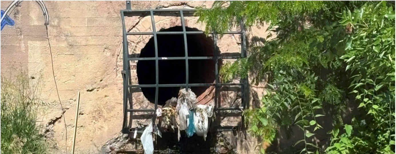
Photograph 11-5. A grated outlet poses a risk to those that enter the storm drain and requires more frequent maintenance. Evaluate all risks and place grates on an outlet only as a last resort. Photo courtesy of City and County of Denver.
