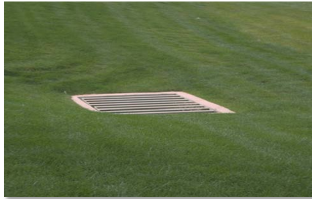
Photograph 7-8. Inlets frequently need maintenance.
