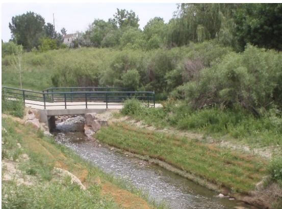
Photograph 8-15. Soil lifts used to stabilize banks of low-flow channel. Photo taken immediately after construction.
