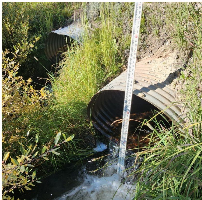
Figure 5: Culvert Perched Approximately 18 Inches
