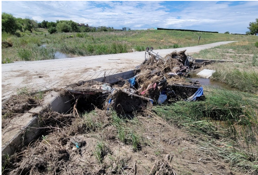
Figure 3: Debris Accumulation at the Entrance to Undersized Trail Crossing Resulting from Storm Event
