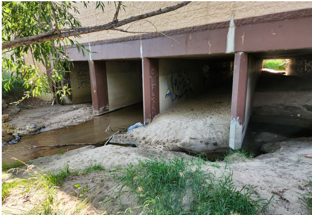
Figure 4: Sediment Deposition at Over Widened Box Culvert
