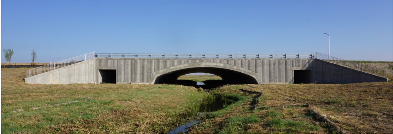
Figure 18: Constructed Crossing of First Creek at E. 26th Avenue in Aurora, Colorado
