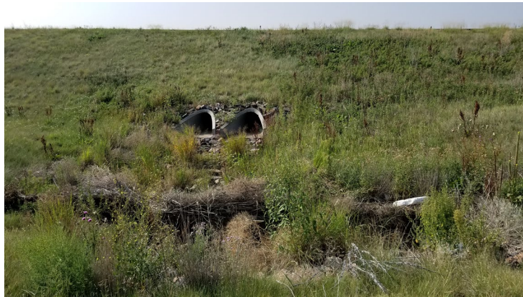
Figure 16: Pre-project photo of First Creek Crossing Structure at E. 26 th Avenue in Aurora, Colorado
